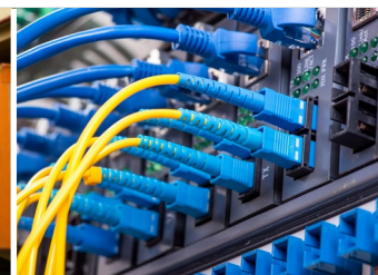
Computer servers and data storage devices
