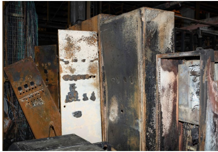
Small-Scale, Isolated Fire Event (Electrical Cabinet)
