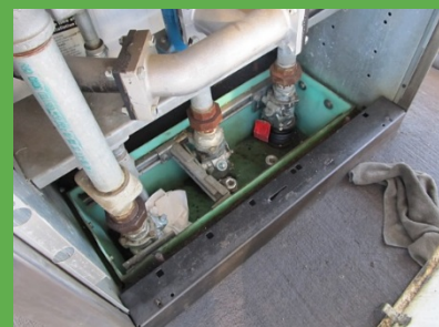
Under dispenser containment
